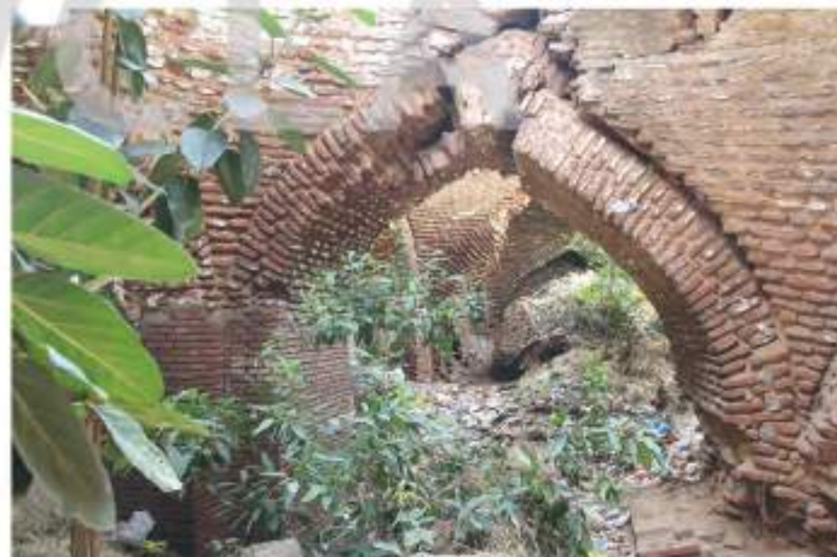
Dilapidated arches of Royal Kitchens
