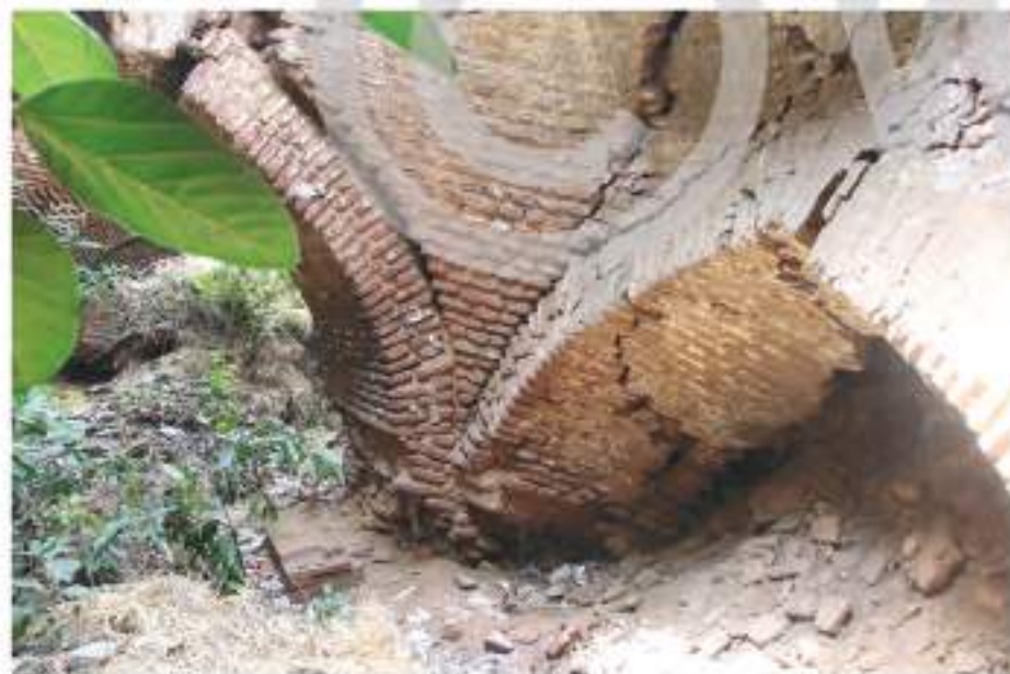
Arches fallen apart inside Royal Kitchens
