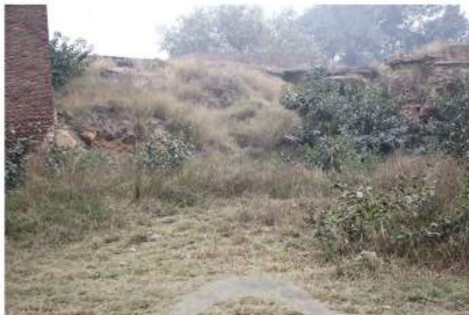
Wild plantation and collapsed structures
